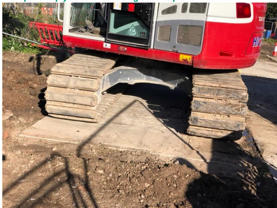
Example of a plywood sheet being used to prevent contact with infested soils
